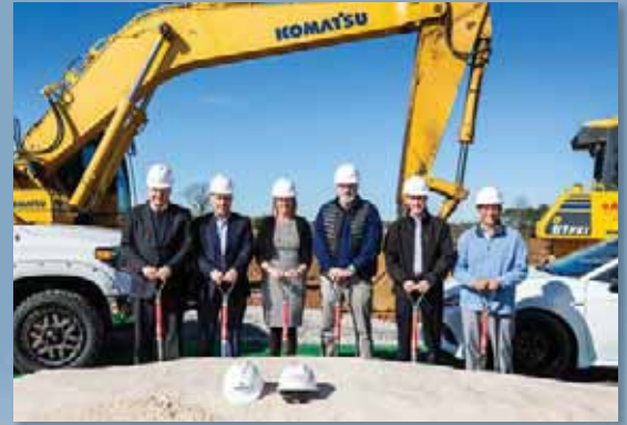
Breaking ground at our new Commerce facility are (L to R): Colin Brown, Brent Burns, Cindy Patterson, Ed Sheehy, Kevin Fleeger and Ray Natour.
